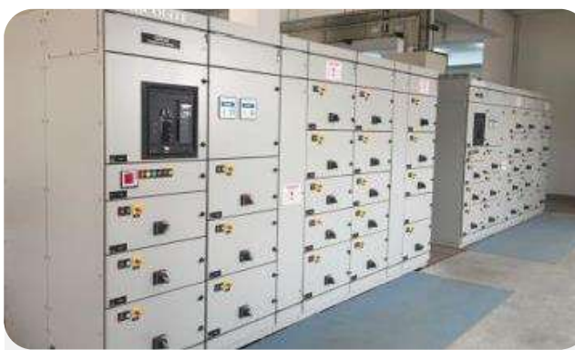
I.T Panel in ESS1 & ESS2
