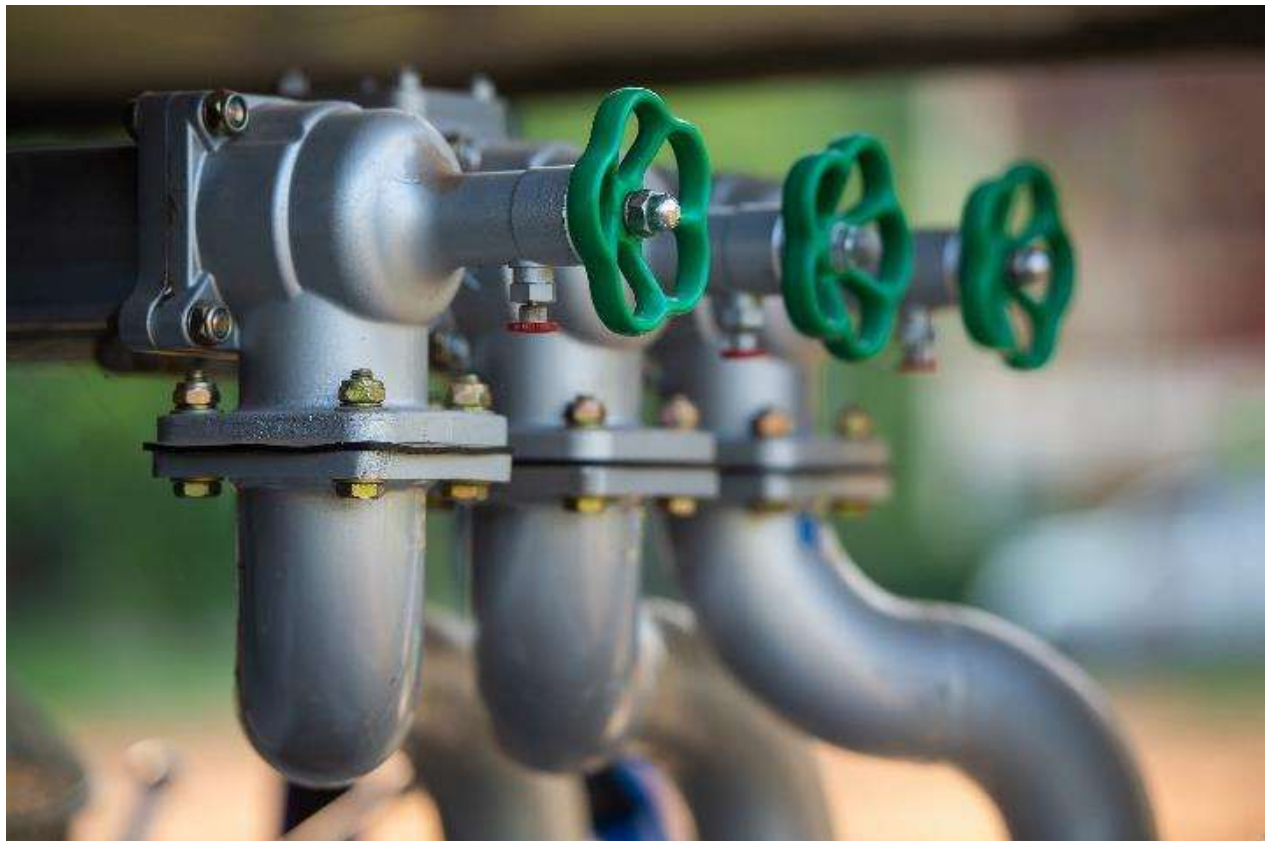
Single Headed Hydrant Value
