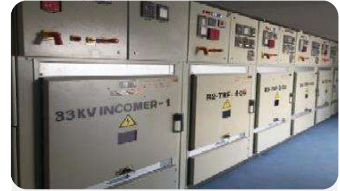
33 KV Panel Main panel & ring panel 2 I/C to 6 O/G Nos.
