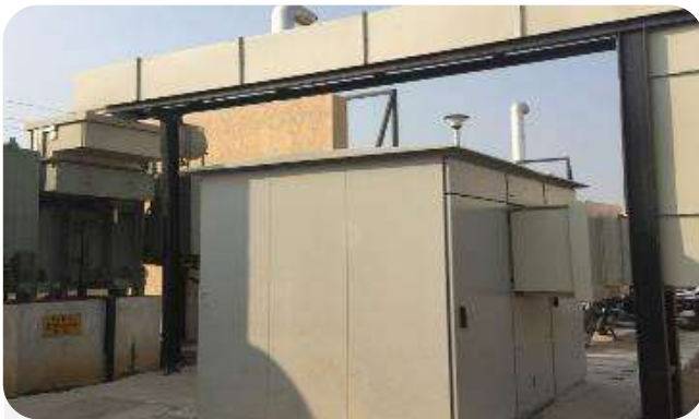
Transformer - 2.5 MVA & 2MVA - 6 Nos
